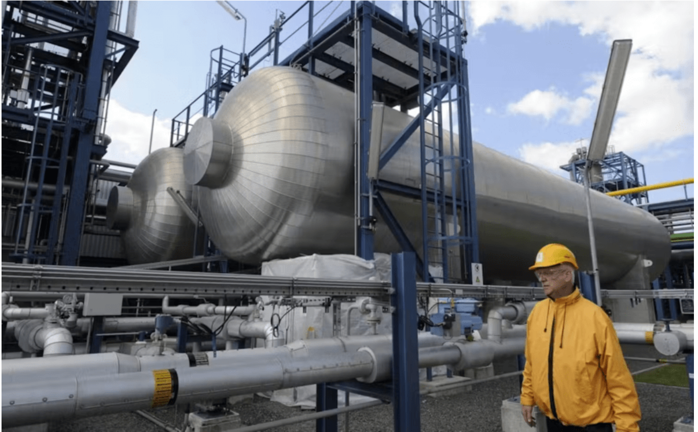
A carbon dioxide capture and storage facility in Brandenburg, Germany, in 2011. The €10m project is a joint venture between Swedish energy company Vattenfall Europe and the US company Air Products. EPA/BERND SETTNIK
